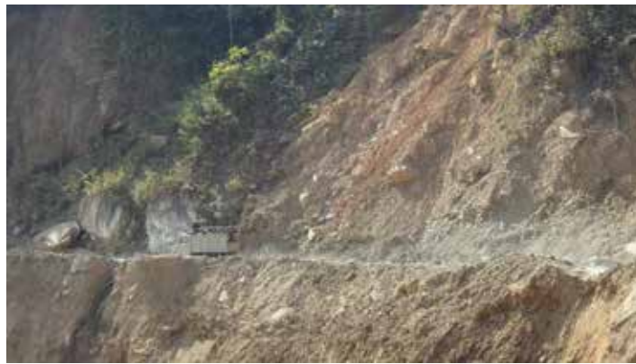
Figure 9 Loose unconsolidated overburden mass in the excavated slope
