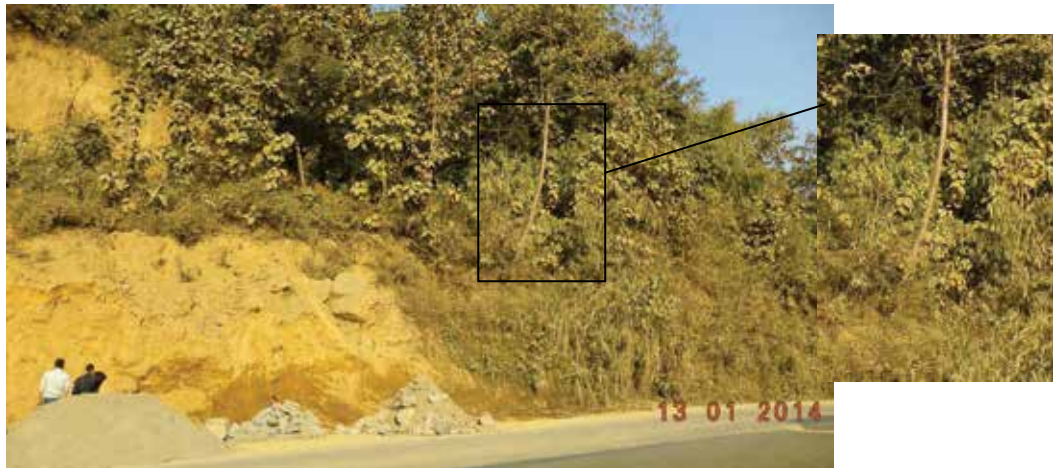
Figure 14 Rotational failure in the cut slope near Mama Cement Factory (Identifiable creep movement in the adjoining slope evident from bending of tree trunk)
