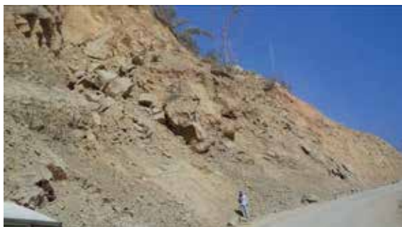
Figure 7 Fragmented and powdery rock mass exposed
