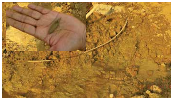
Figure 12 Prominent seepage and clay deposition in the basal overburden slope (Inset shows deposited moulded finer material)
