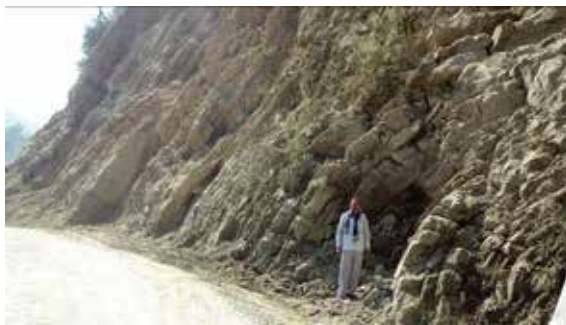
Figure 5 Steepening of the dip and seepage of water
