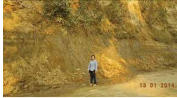
Figure 11 Extensive damp patches in the exposed rock mass as observed during dry period
