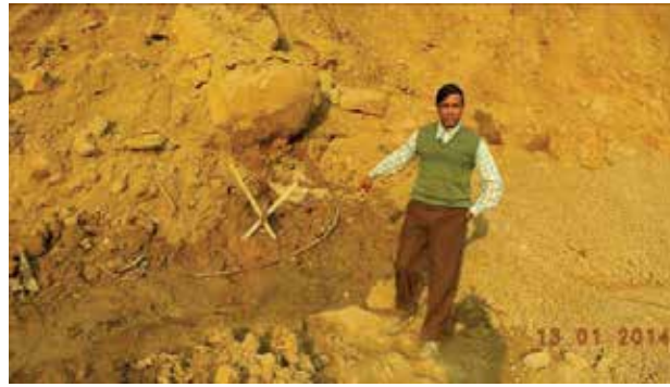
Figure 4 Seepage of water in the loose overburden
